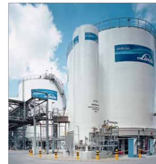
Linde Gas's biggest European gas centre is located at Leuna Chemical Industry Park – and supplies customers throughout the region
