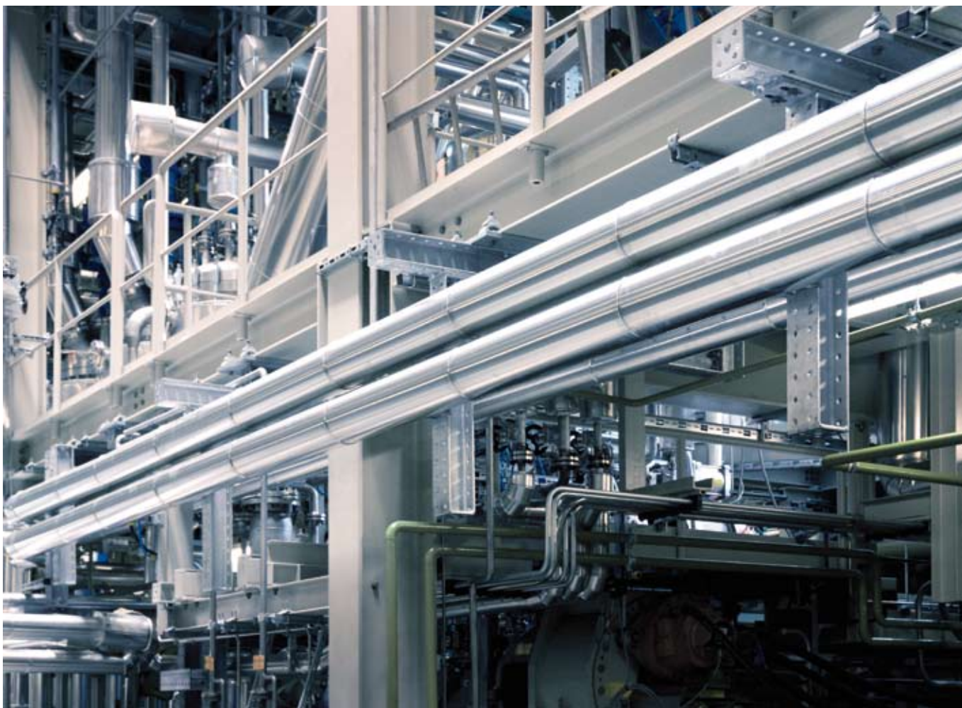
Fraunhofer pilot plant centre for polymer synthesis and processing Schkopau PAZ
